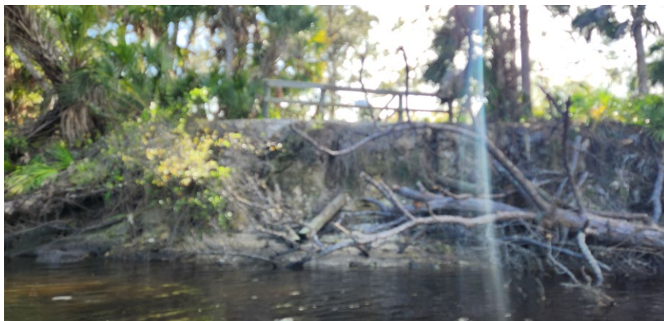
Activities near the southern overlook at the Venetian Golf and River Club may have caused additional bank failure since the last inspection.
