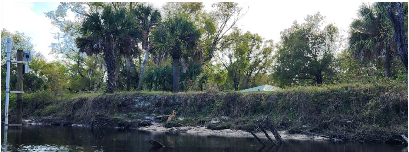
This area along VMRP where the bank has experienced some annual erosion. This bank is near a multi-use recreational trail. Some discussions have occurred about moving the trail and/or attempting to stabilize the bank with natural materials and plantings.
